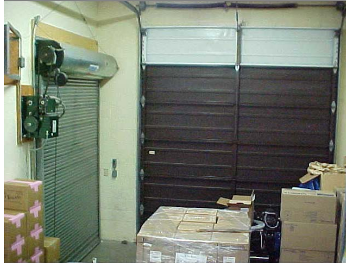
Figure 23 Typical cargo bay, with metal coiling slat door (similar to Specimen #5) and a non-insulated sectional garage door (similar to Specimen #1)
